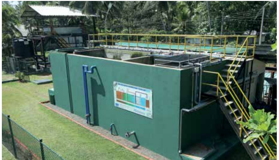
Membrane bioreactor effluent treatment plant at CCS Ranala factory
