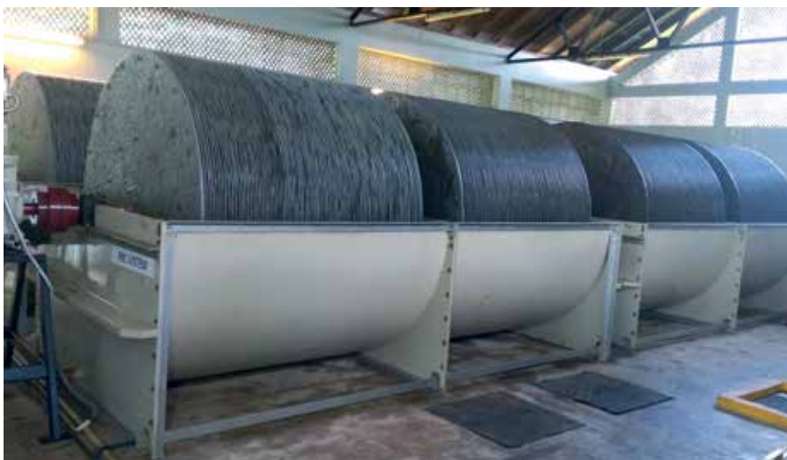
Sewage treatment plant at Cinnamon Bay
