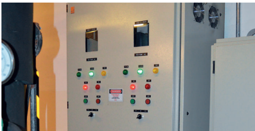
Variable frequency drive (VFD) panels installed at Cinnamon red
