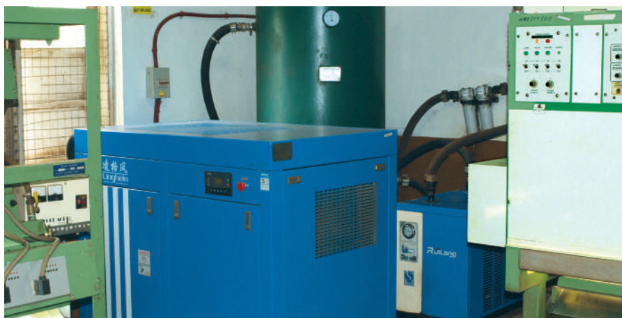
Energy saving screw compressor installed at Neluwa Medagama tea factory
