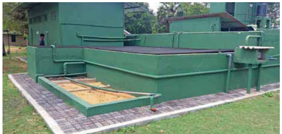
Sewage treatment plant at "Trinco Blu by Cinnamon"
