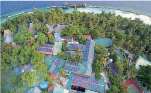
Solar photovoltaic system installed at "Ellaidhoo Maldives by Cinnamon"
